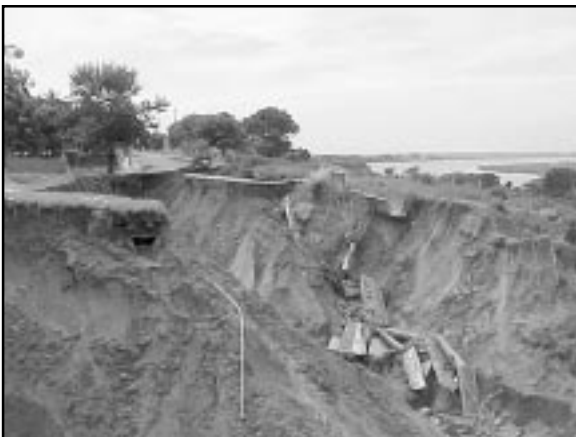
Flood damaged road
